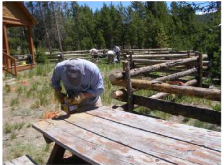
Digger sanding a table at Redfish lake project. Crew in the background painting another table after the fence was finished.
