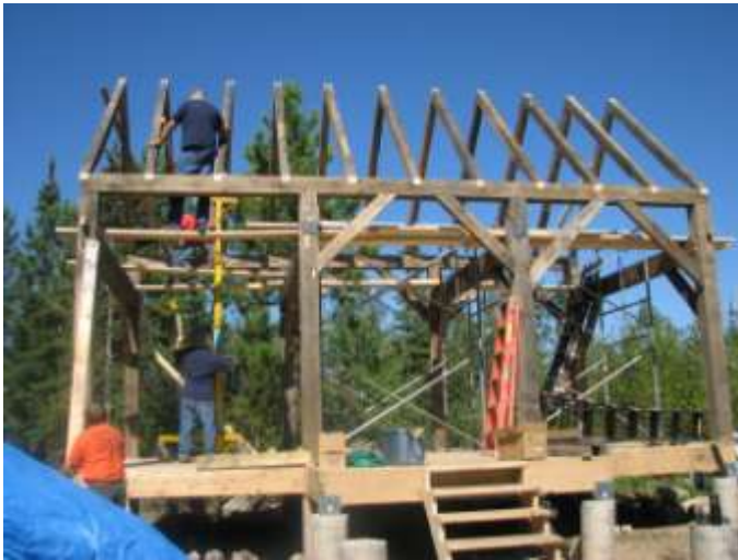
Timber framing top to bottom: Don Havel, Peter Henrickson, Bob Aldrich, Don Larson
