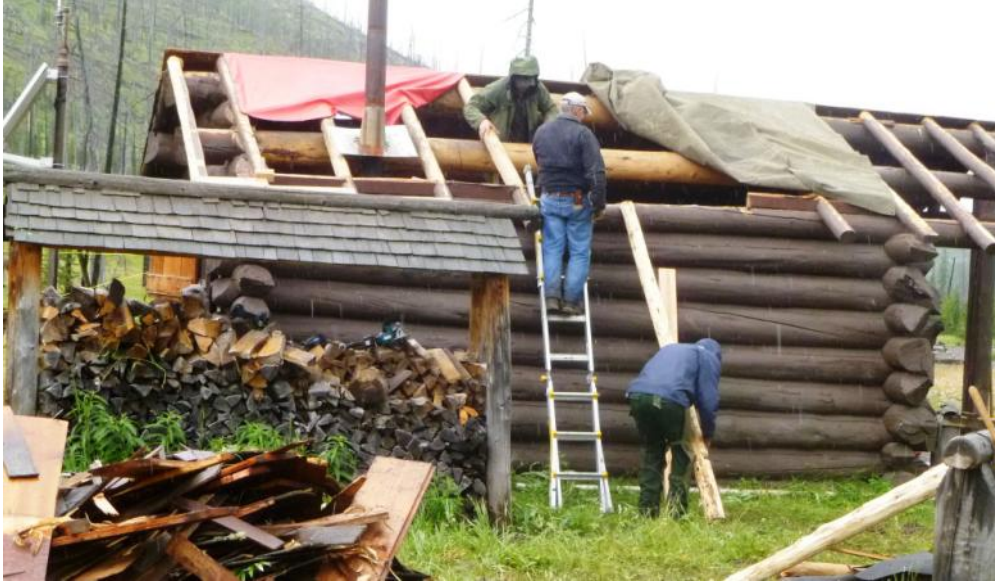
Setting perlings- Gabe Gassman (top), Jack At- kins on the lad- der, Don Whyde on the ground
