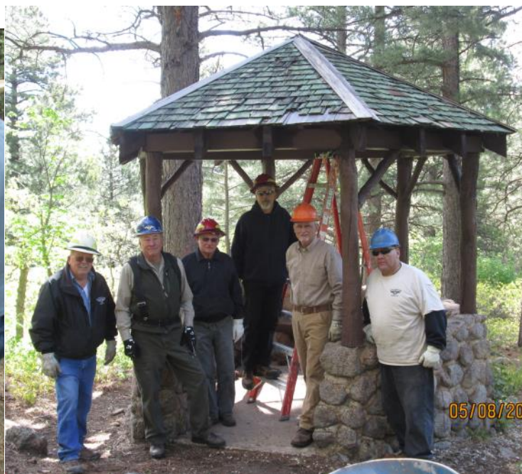
Crew at old Gazebo before starting work. L-R; Digger Daniels, Doug Wamsley, Jim Rush, Tom Wilkes, Gary Johnson, and Chuck Orona.
