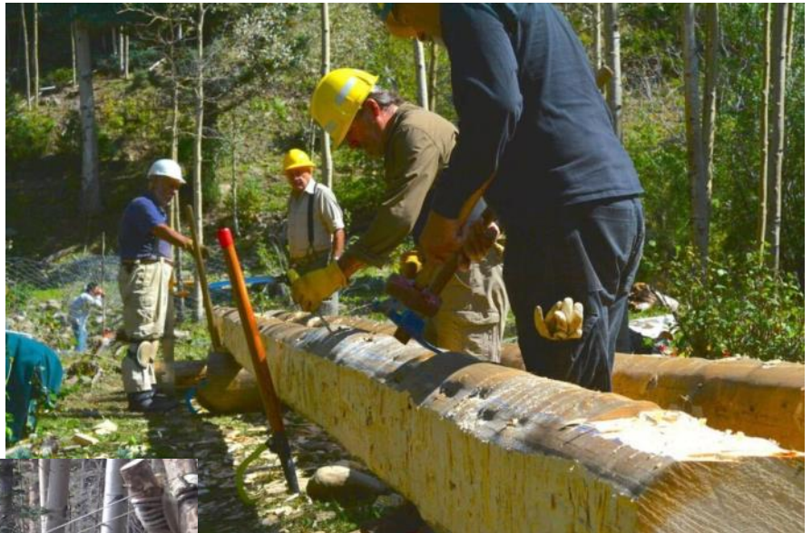
Jumpers working on a stringer for the bridge. Photo by David Barager
