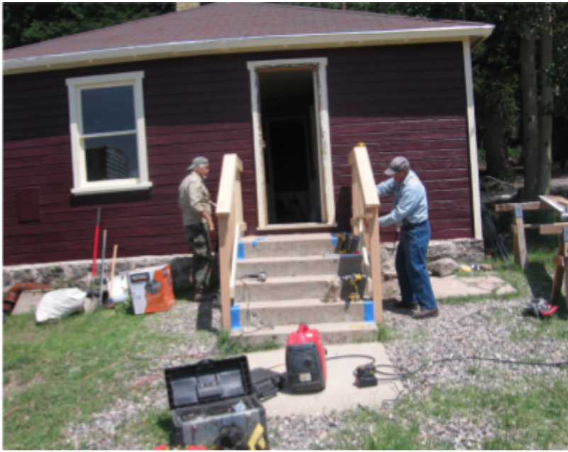
At the Ranger Station (L-R): Tom Wilks and Scott Warner working on the railing for the porch
