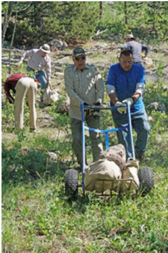
(Left) Ryan Siple and Ben Robinson (Park Service) deliver a load of rocks and position rocks to lock bridge supports
